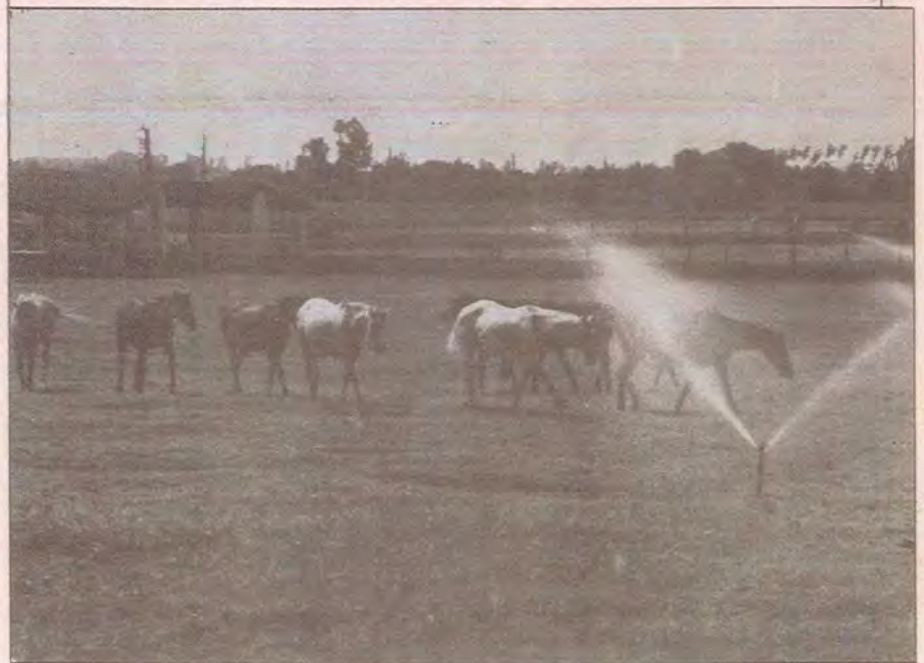
Automatic Pop up Sprinklers with complete underground pipes
